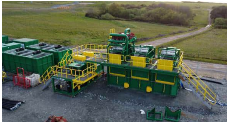
Figure 6.5: Drill Fluid Recycling Plant (typical)
